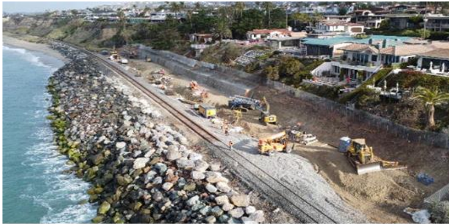
4. Impacts of erosion of bluffs along the LOSSAN Rail Corridor
